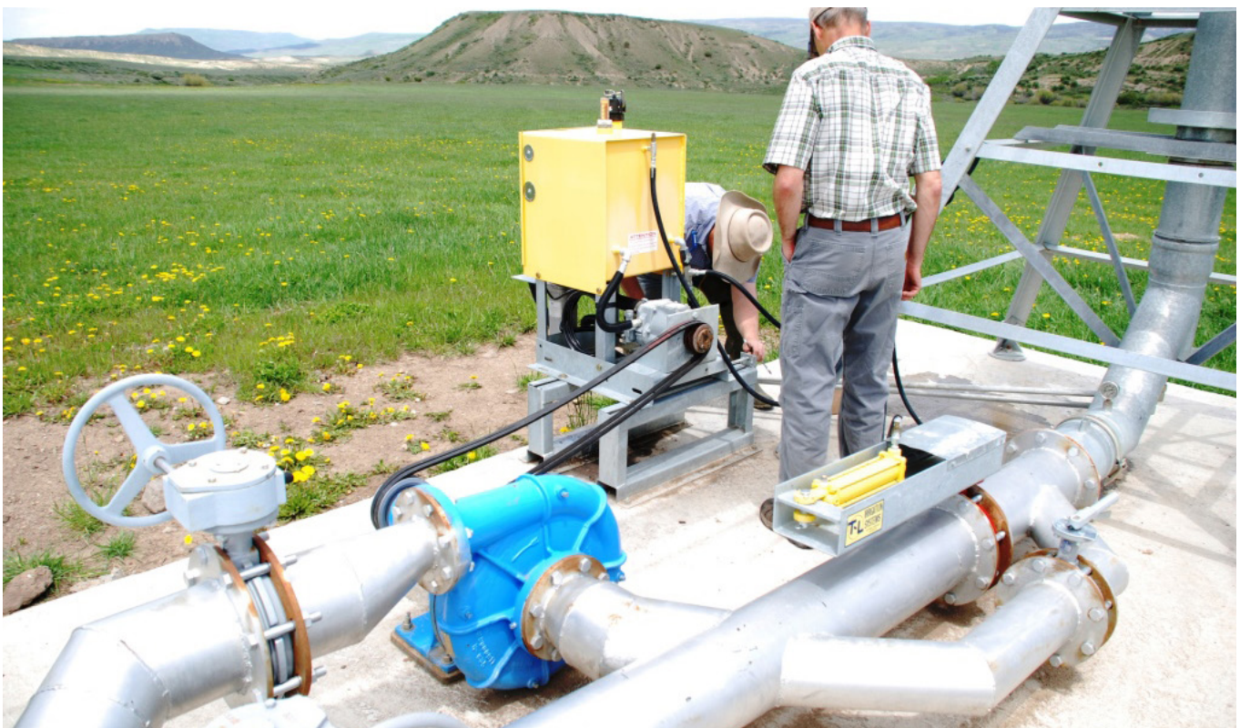
The first joint project to help farmers use existing irrigation water to generate electricity has been completed near Hotchkiss, Colorado. Photo by Sam Anderson, Colorado Department of Agriculture.
